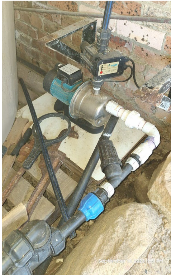
Electric Pump Under House
